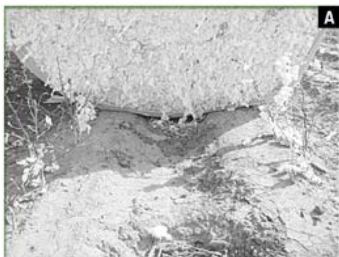
Incorrect Staging Surface
